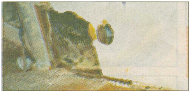
ROTTEN MESS: Leaks have rotted the timber framing of Malcolm Fort's garage.
